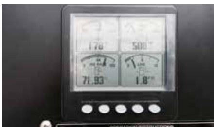
Dual fuel system operating showing gas use percentage at 71.93% and diesel use at 1.8 gallons/hour (same load).
