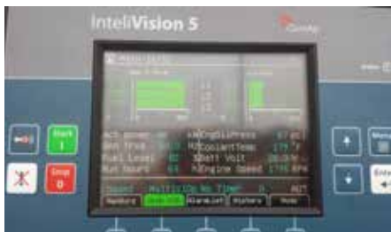
Parallel Control Module showing current load (46Kw).
