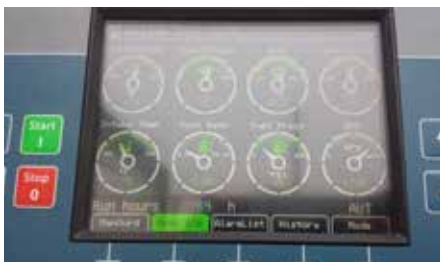
Parallel Control Module showing current diesel use while running in HDF mode.
